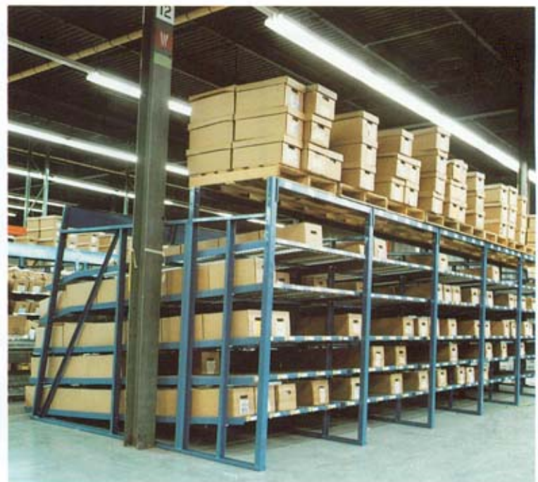
Restocking side of Keneco system. Single level pallet storage is provided above.
